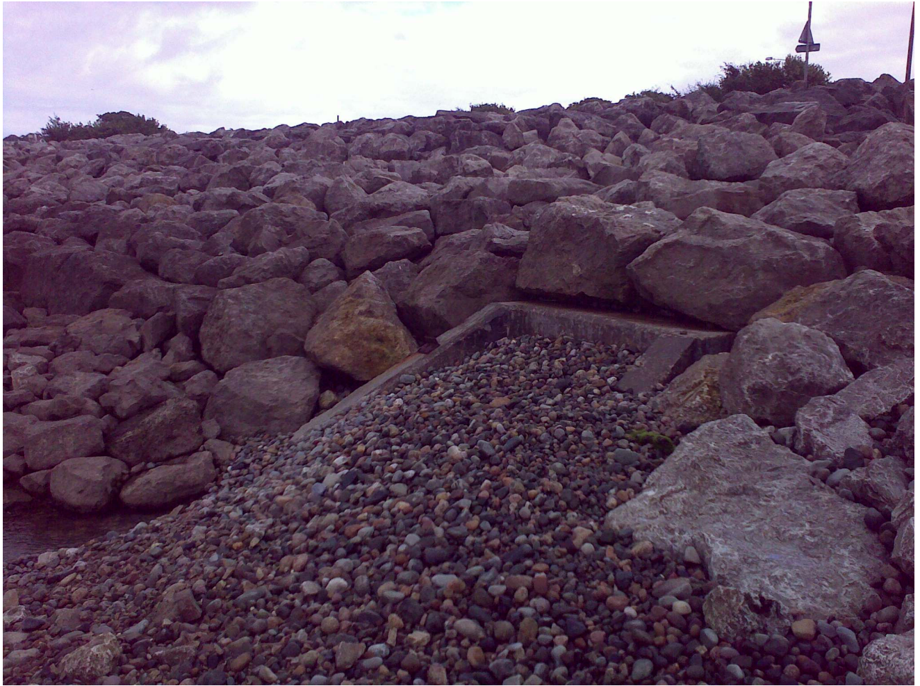
Outfall when blocked with 8 tonnes of shingle after a spring/ rough high tide.
